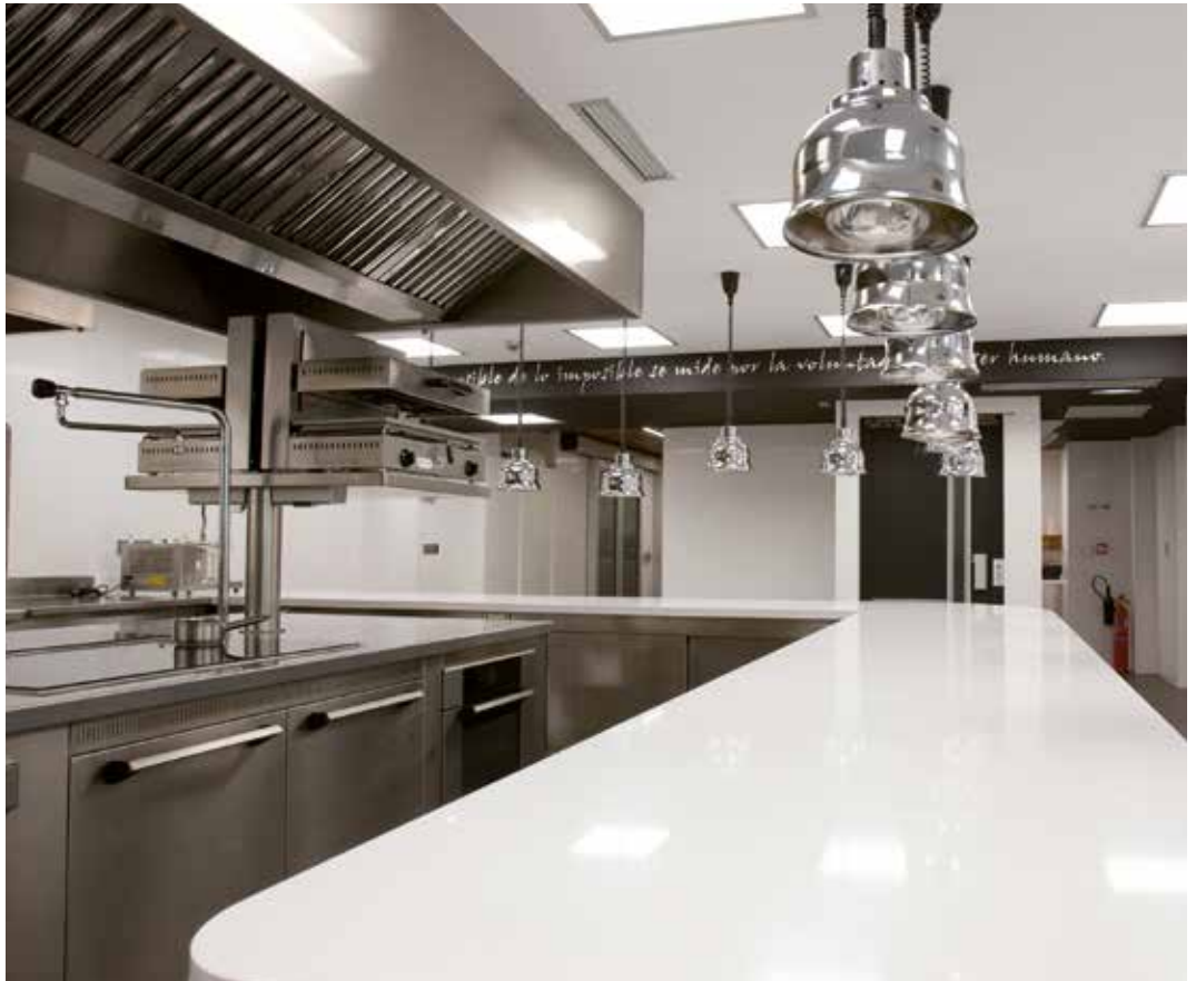
KÜCHE RESTAURANT MUGARITZ / CUCINA RISTORANTE MUGARITZ
