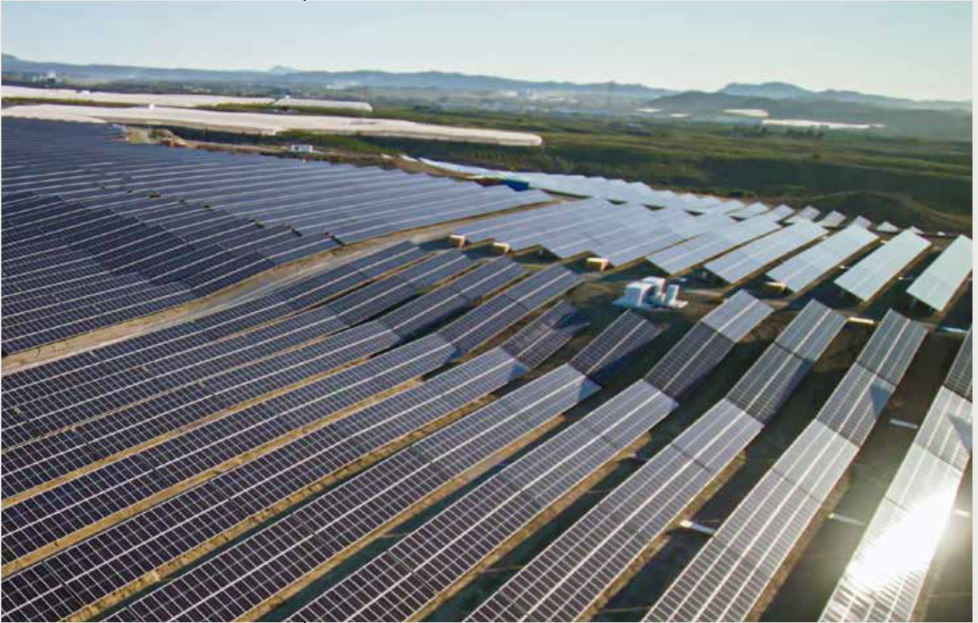
Photovoltaic solar plant at Cosentino industrial park in Almería, Spain.
