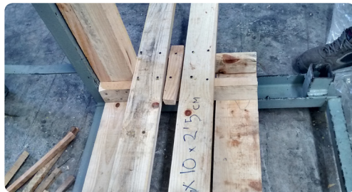
Step 2: Securing the planks to the base (see detail in the following photo).
