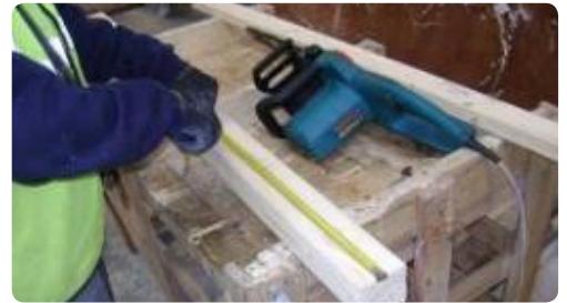
The planks are cut to size: between the pallets and between the pallets and the walls of the container.
