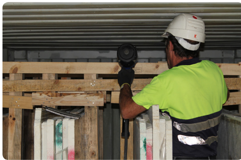
Firstly, long planks will be laid that touch the sides of the container, to join the highest number of pallets together.
