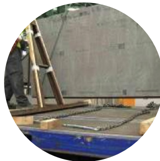
Repositioning part of the rack before finally depositing the load (to ensure its correct seating).
