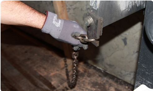
The auxiliary operator will pull the chain and centre it.
